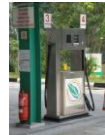
CNG Compression & Dispensing 天然气压缩&加注
